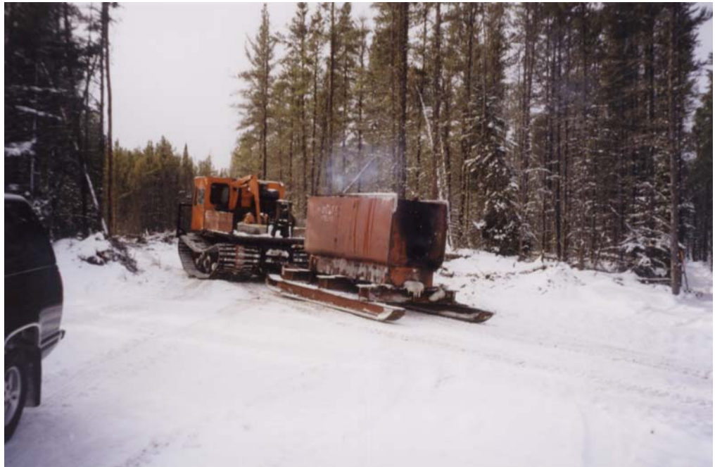
Plate 7: Other heavy equipment involved in mineral exploration – water en route to drill site.
