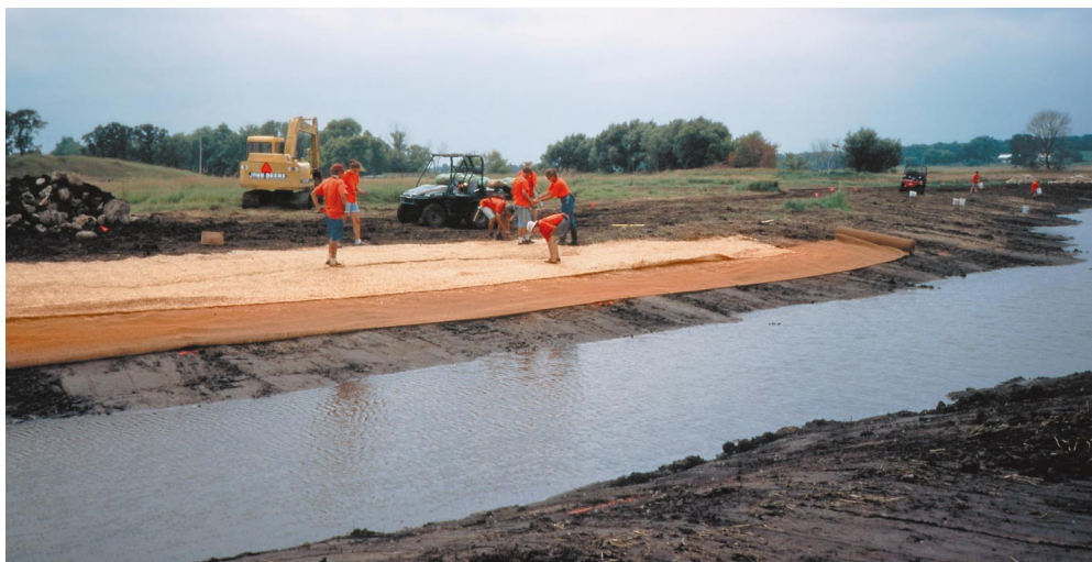
Fig. 1. A 2.6 km segment of Nippersink Creek, Illinois, USA, was filled in to make farming more efficient. Here, the meandering creek is being restored by excavating the historical channel, contouring the banks, anchoring mats to control erosion, adding a mulching blanket and seeds to encourage native vegetation, and planting propagules of aquatic plants. The project has multiple goals: reduction of flooding downstream; improved water quality; habitat for fish, wading birds and waterfowl; and involvement of youngsters in the process (Ed Collins, project director and restoration ecologist with the McHenry County Conservation District, pers. commun.). Photo by J. Zedler.
